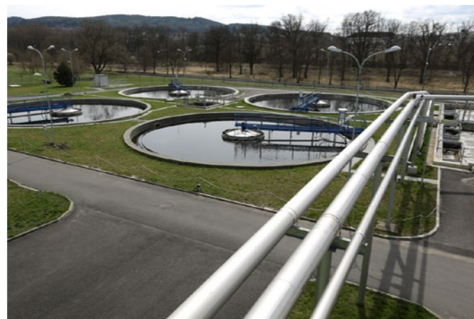
Wastewater treatment plant Strakonice (75 000 inhabitants)
